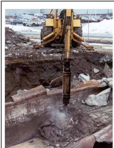
Whether it be getting a difficult tank out of the ground or remediating a release, ECL can help.
